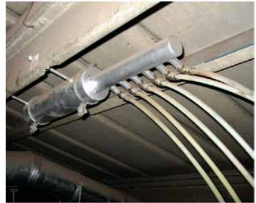
Figure 21 Multiple air exhausts piped to a manifold and silencer
