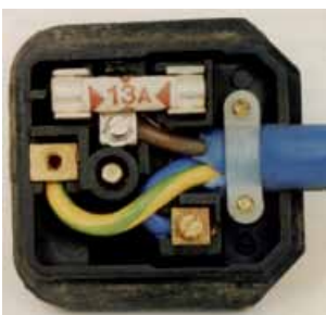
Missing screw on earth connection
