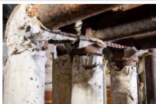
Asbestos insulation on pipes
