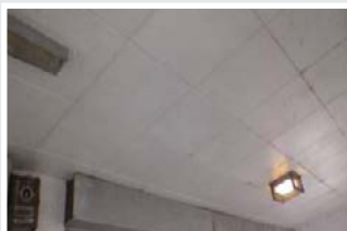
Asbestos insulation board ceiling
