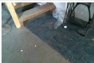
Vinyl floor tiles containing asbestos
